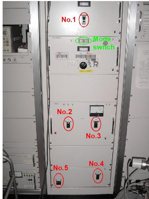
Control Panel of the New Calibration System
